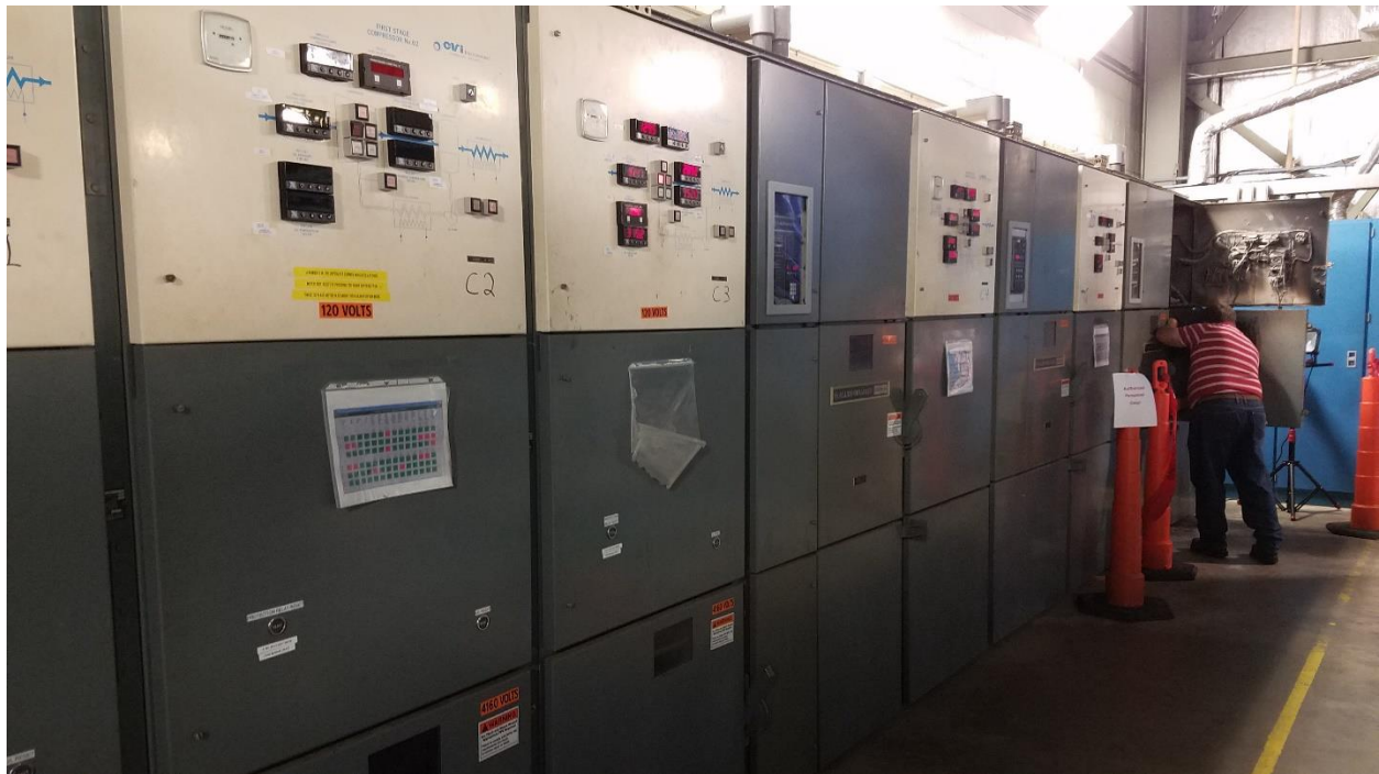
Figure 1 The entire bank of motor control center starters for the 2250HP compressors in the building
