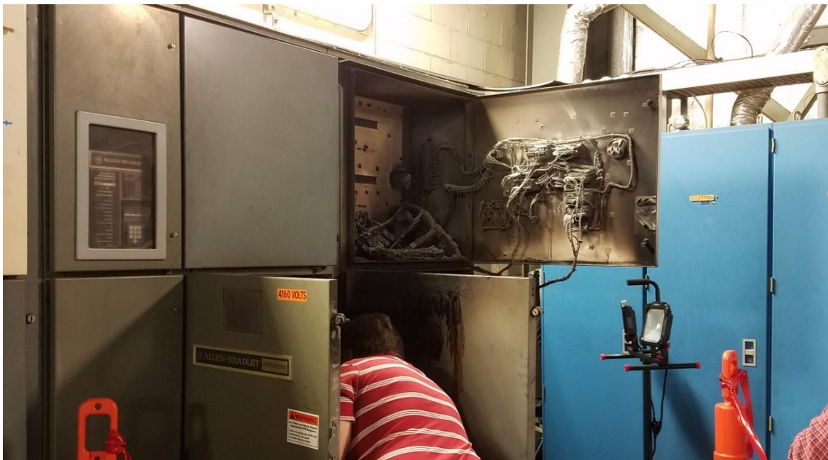
Figure 2 - Compressor 6 MCC – cabinets left to right, PMP, contactor/fuse, and autotransformer.
